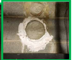
Capped emissions vent
